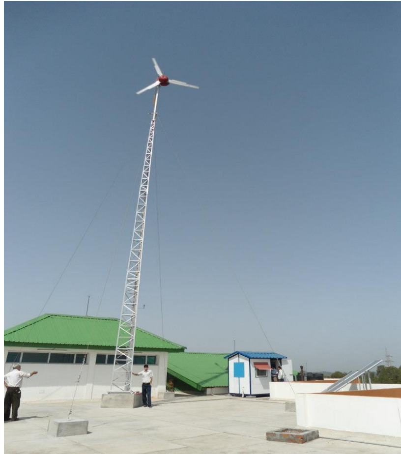
Fig. 4.10 Solar-wind-battery hybrid system installed at CEE, NIT Hamirpur
