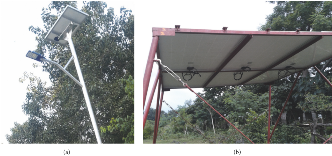
FIGURE 2: Solar street lamps for (a) farm lighting and (b) the 6-panel PV installation.
