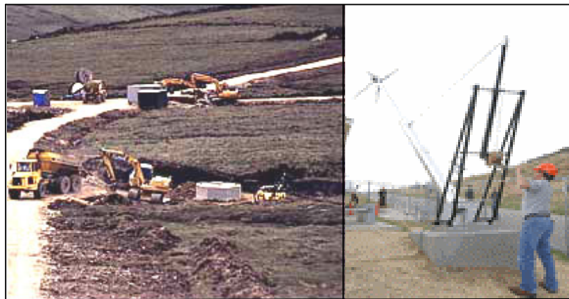
Figure 16: Left; Novar Wind Farm, Scotland, under construction in a moor, July 1997. Right; a man is using mount/crane to lift turbine to operating position.
