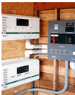
Figure 18: Inverter and controllers at Bullard, Kent - National Park Service
