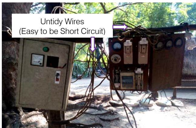
Fig. 13: Distribution Board of Mini-Grid
