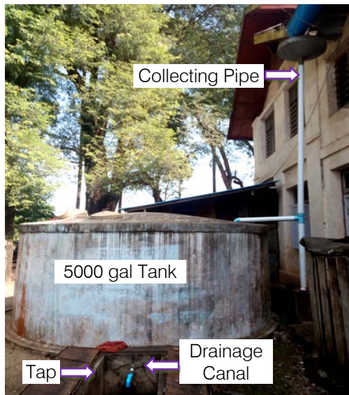
Fig.15: Rain Water Storage at the Monastery
